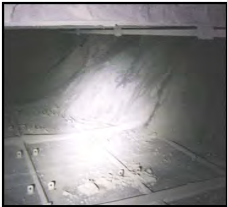
Unit 2 – 2 nd Catalyst Layer Ash Pile along the Front Wall
