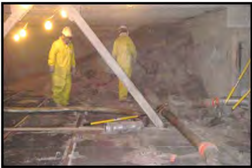
The ash piles were vacuumed during the outage at great expense.
