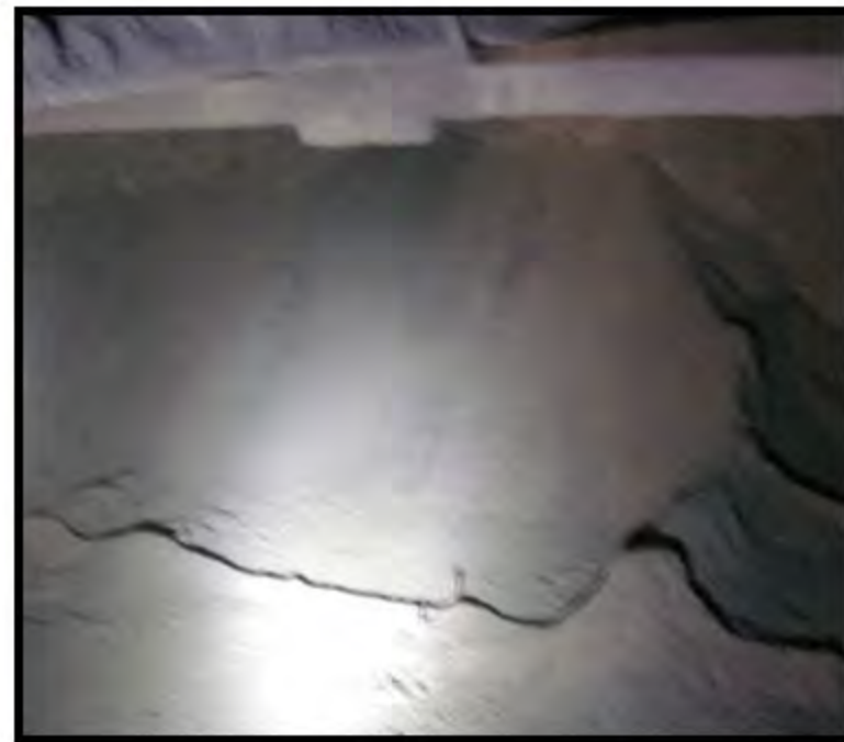
Unit 1 – 3 rd Catalyst Layer Ash Pile along the Rear Wall
