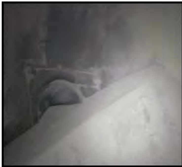
Unit 1 – 1 st Catalyst Layer Ash Pile along the Front Wall
